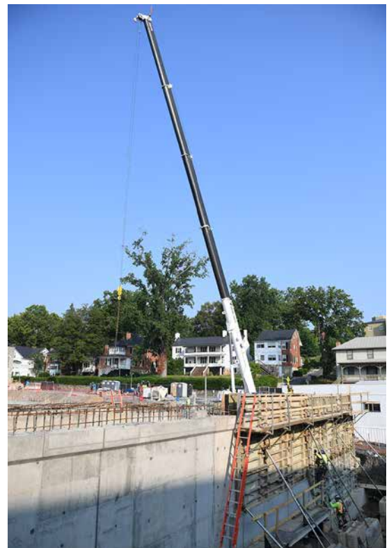
Construction continues on the Aquatic Center, which will contain an indoor 50-meter swimming pool, two 1-meter springboards, two 3-meter springboards, and a 5-meter dive platform, plus seating for 570 spectators.—VMI Photo by Kelly Nye.
