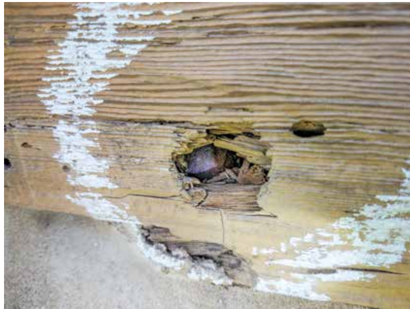
3-inch Hotchkiss canister shot embedded in the wood beam.
